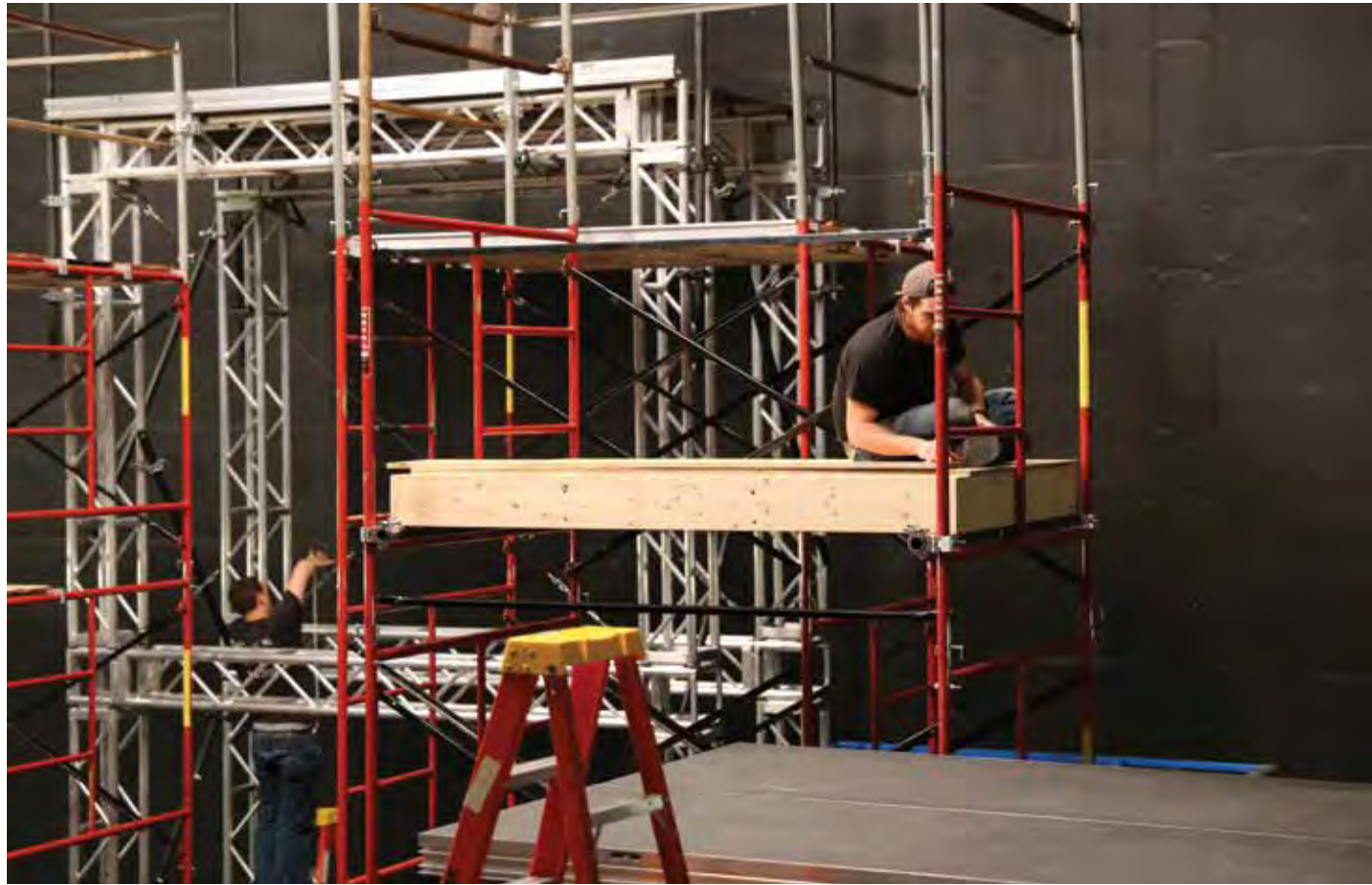
SET CONSTRUCTION FOR A FILM SHOOT IN THE THEATER ( NO FOOD, NO MONEY, NO JEWELS , SUSSMAN/LEE, 2014).
